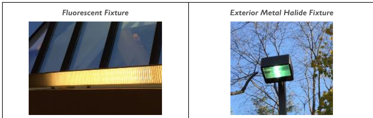
Figure 9 - Building Lighting Systems
